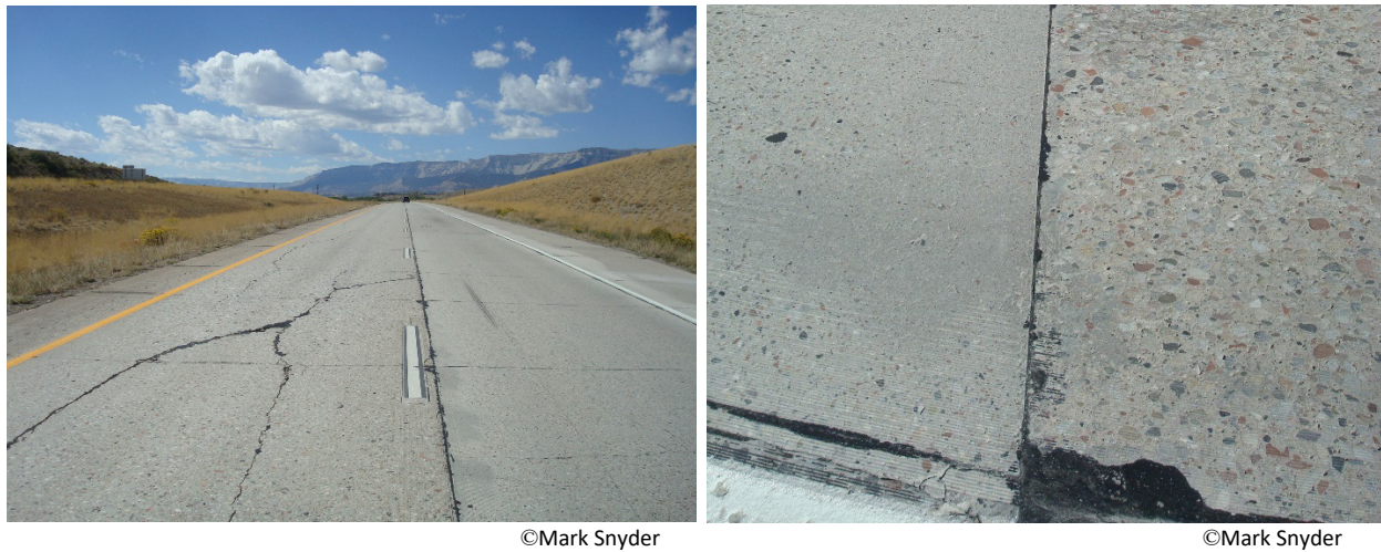
Figure 10-12. Examples of visible concrete color and aggregate size differences between original pavement and full-depth repairs.
