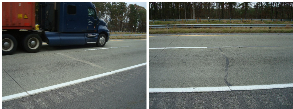
Figure 5-8. Typical 2018 mid-panel transverse cracking with different amounts of partial-depth spall repair.
