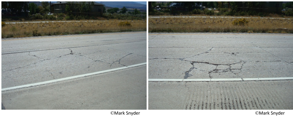
Figure 10-13. Examples of shattered slabs.
