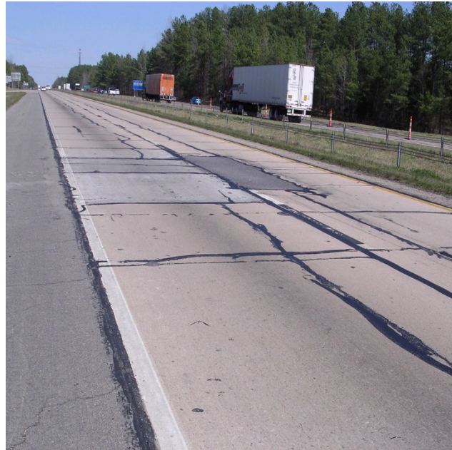
Figure 5-2. Typical CRCP condition prior to overlay in 1997 (source: Morrison 2017).
