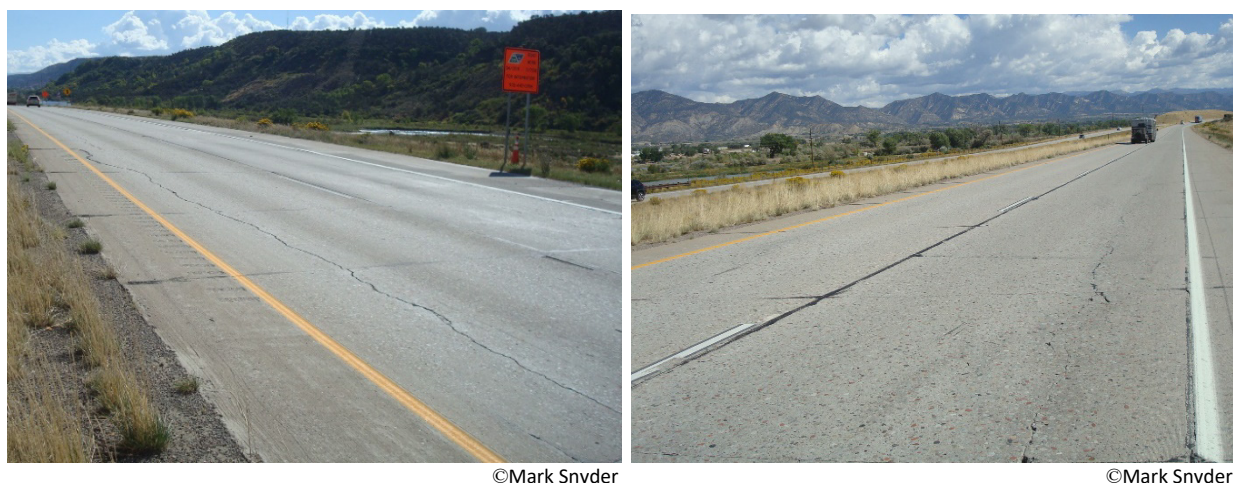
Figure 10-9. Examples of typical longitudinal cracking in the inside lane (left) and outside lane (right).
