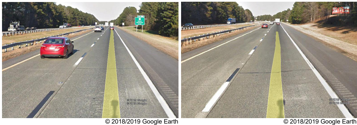
Figure 5-7. Typical 2018 mid-panel transverse cracking with only joint sealant applied (source: Google Earth, December 2018).
