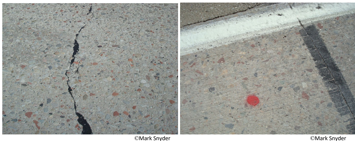
Figure 10-11. Examples of typical surface texture in original pavement (left) and replaced panels (right).
