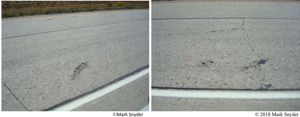
Figure 10-15. Examples of displaced rebar at pavement surface in outer wheel path of westbound driving lane.
