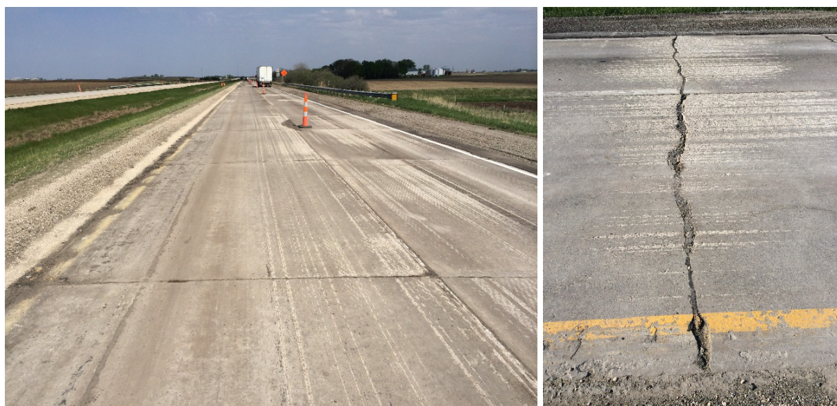
Figure 8-4. Exposed concrete (left), close-up to pre-existing cracking in eastbound direction of U.S. 20 (right).
