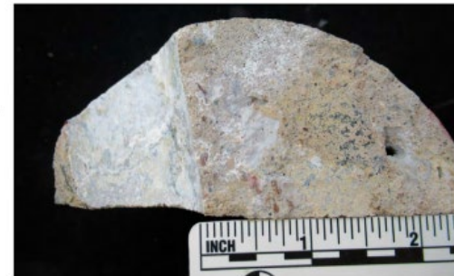
Photo: 10 Sample ID: 62A Description: Corrosion product coating the impression of the dowel bar and extending laterally into the concrete paste, viewed on the bottom surface of the core sample.
