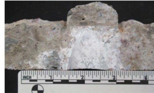
Photo: 9 Sample ID: 62A Description: Corrosion product coating the impression of the dowel bar and extending laterally into the concrete paste, viewed on the sub-horizontal fracture plane of the sample.
