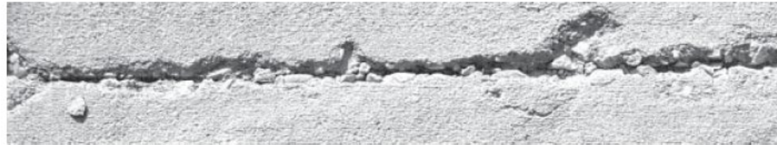
A. UNACCEPTABLE RAVELING - Sawed too early
