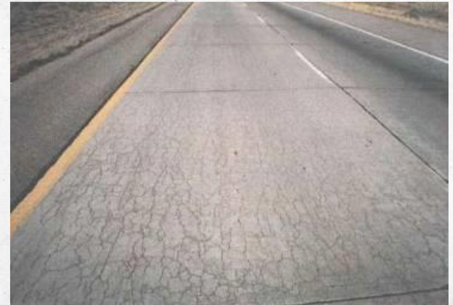
Class F Ash was all that was allowed Thought was—to restrictive
