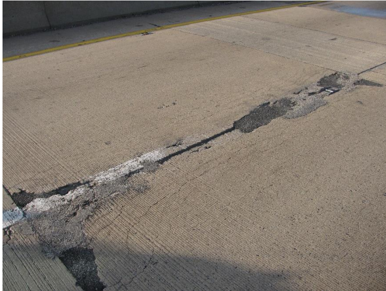
Figure 2. Severe D-cracking in a pavement section in Pennsylvania inspected by the research team
