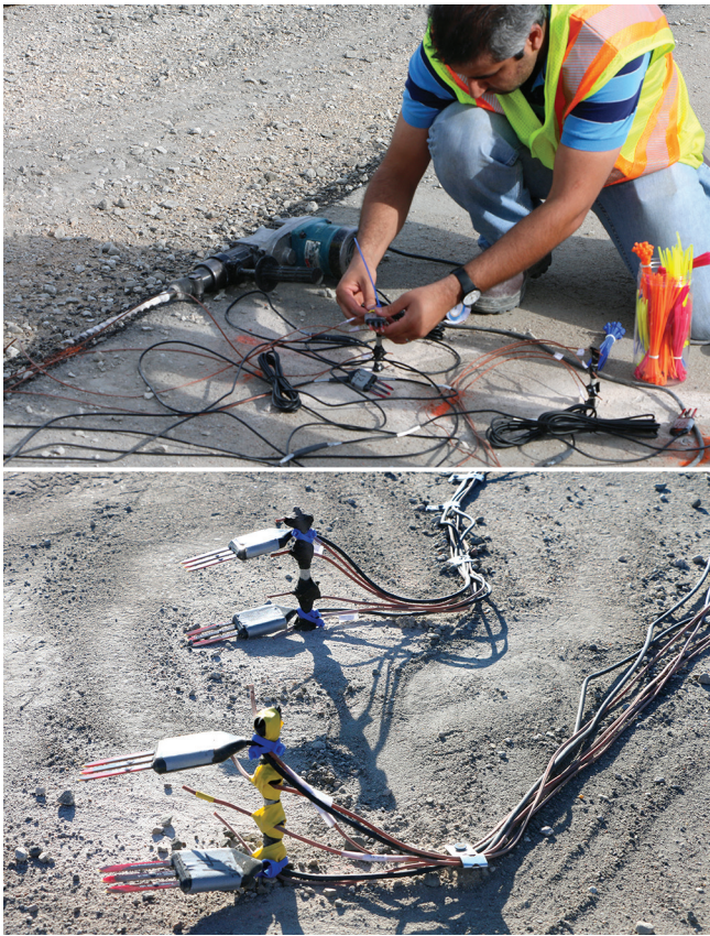
Preparation of wiring for pavement sensors (top) and sensors mounted one inch and five and a half inches above the pavement base (bottom) before overlay paving on Washington County Road W-61
