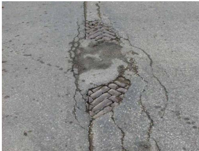
Figure 1. Asphalt surface with exposed brick
