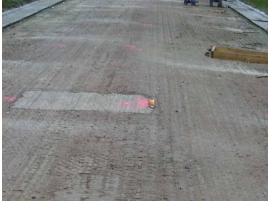
Figure 11. Milled surface and existing PCC patches
