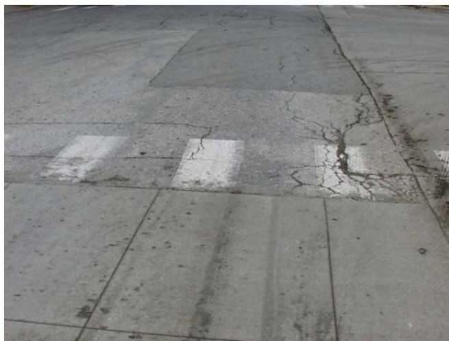
Figure 2. Deteriorated asphaltic concrete surface
