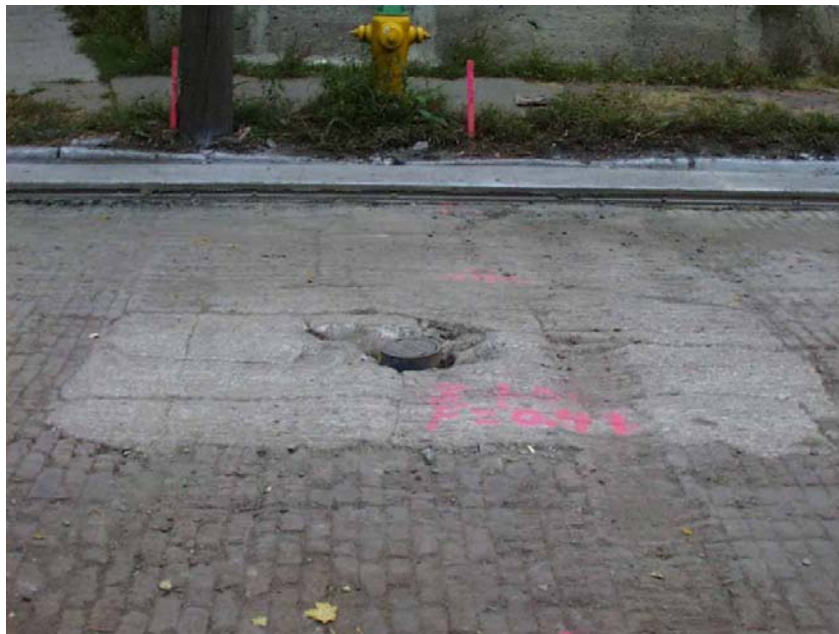
Figure 14. Water valve adjustment area
