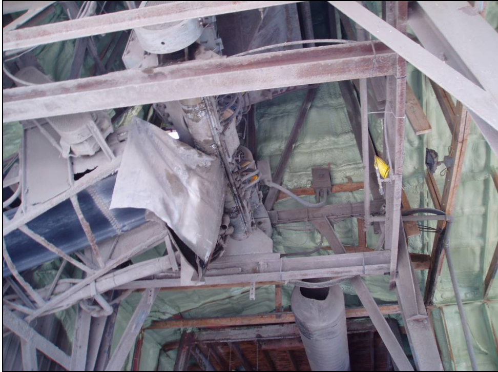
Figure 45. Underneath side of the Hydromix plant
