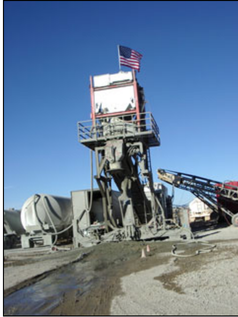
Figure 36. Two-stage mixing plant on site
