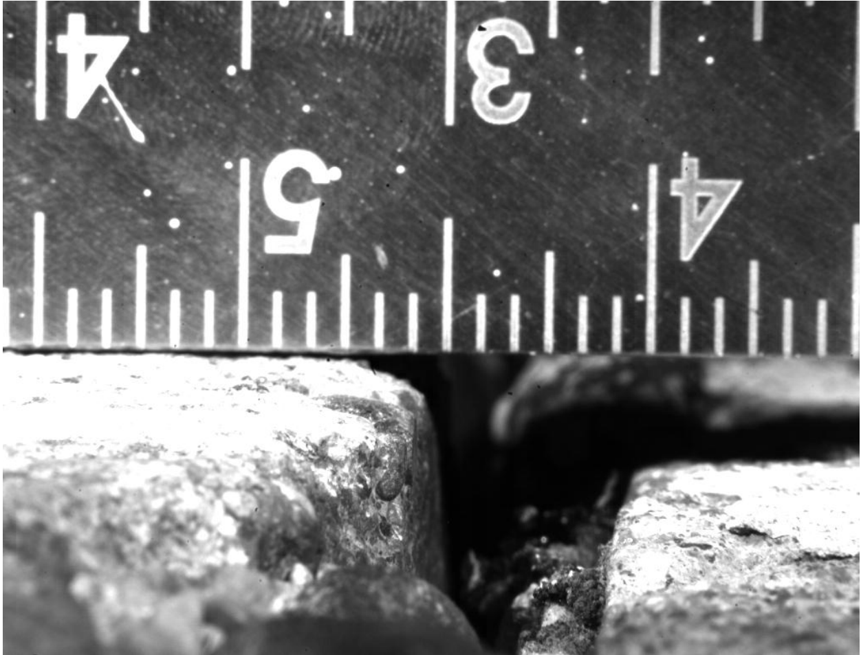
Figure 4.1. Sample still frame from Photron Fastcam® illustrating faulting of approximately ¼ inch
