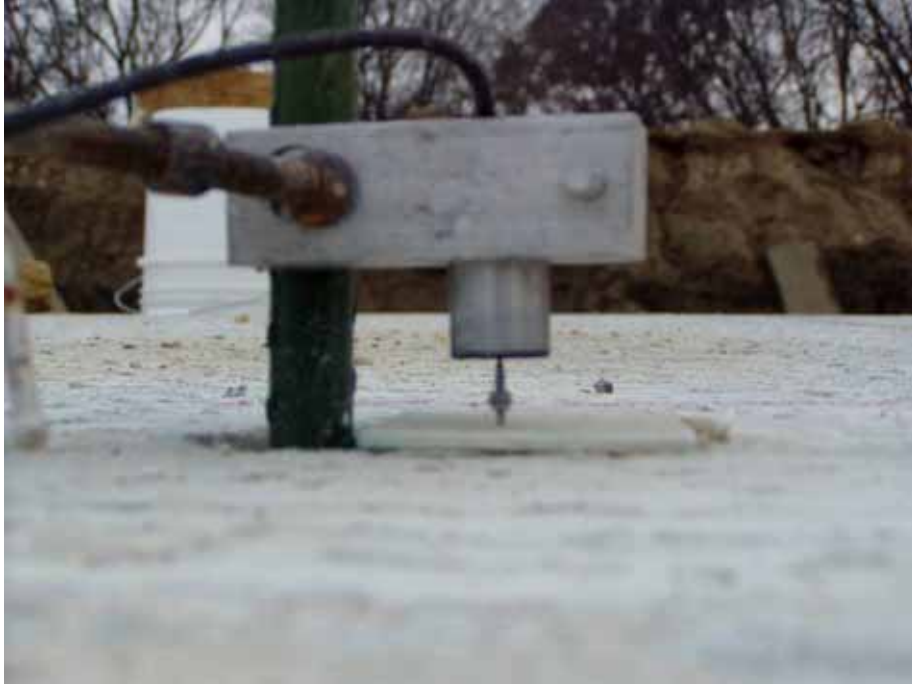
Figure A19. LVDT installation (Iowa State University)
