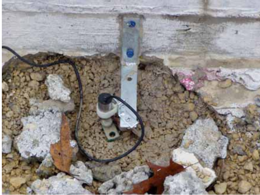
Figure 11. LVDT installation (Transtec)
