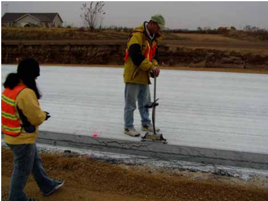
Figure A12. Inclinometer profiling
