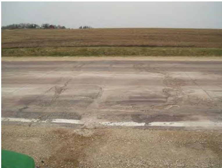
Figure 20. Full-depth patch area with multiple distresses
