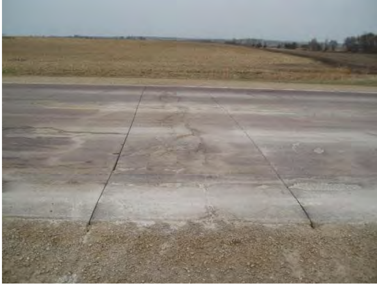
Figure 19. Full-depth patch area
