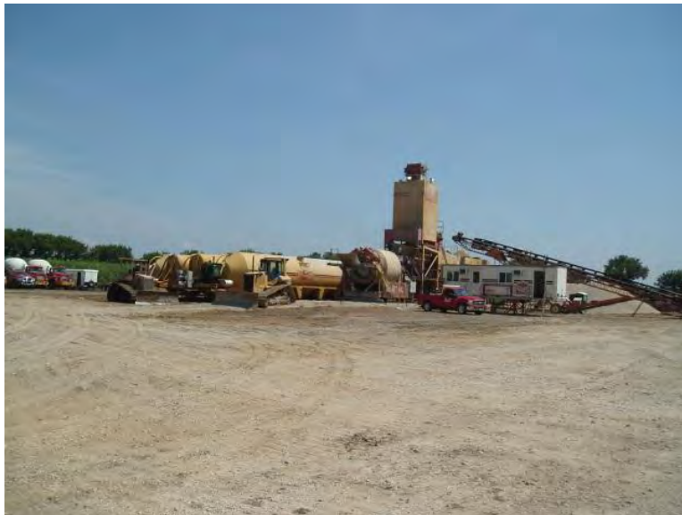
Figure 85. Central mix concrete batch plant
