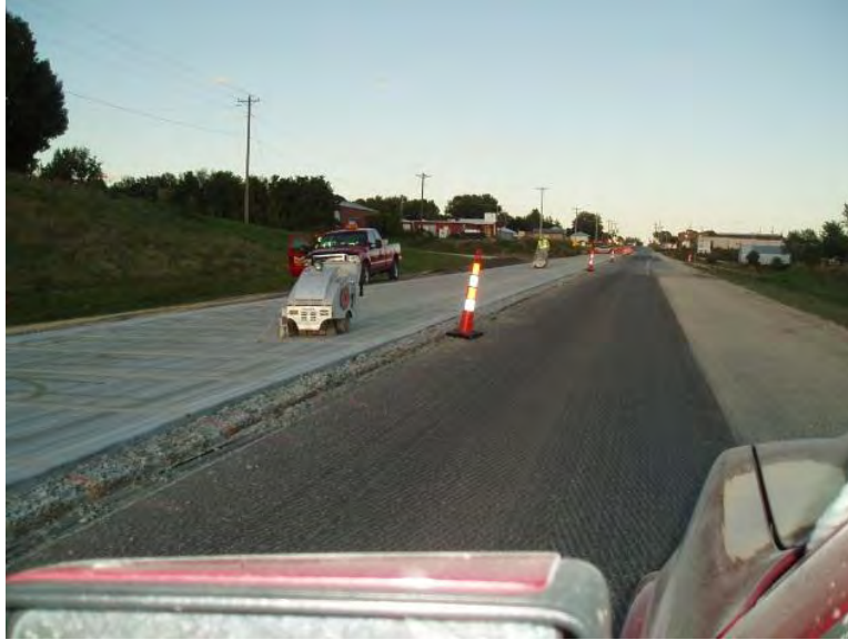
Figure 87. Longitudinal joint saws
