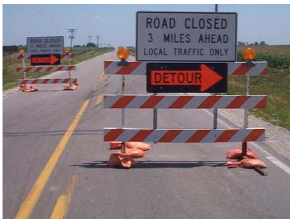
Figure 11. Typical Road Closure
