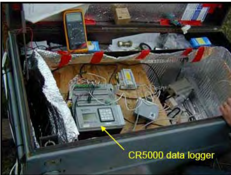
Figure 3-13. Data acquisition system at Pole 2
