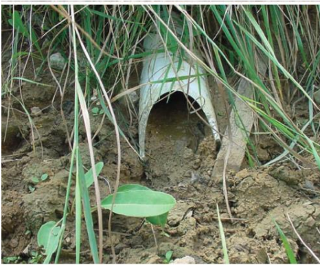
Figure 7. Clogged subdrain outlet (Photo courtesy of Chapter 7, Concrete Pavement Preservation Guide, CP Tech Center)
