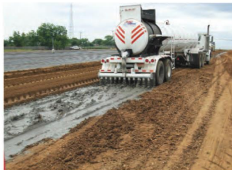
Figure 2. Cement slurry application (Photo courtesy of Guide to Integrated Pavement Solutions, CP Tech Center)
