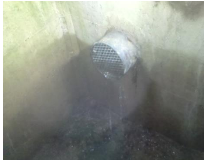
Figure 8. Urban subdrain outlet
