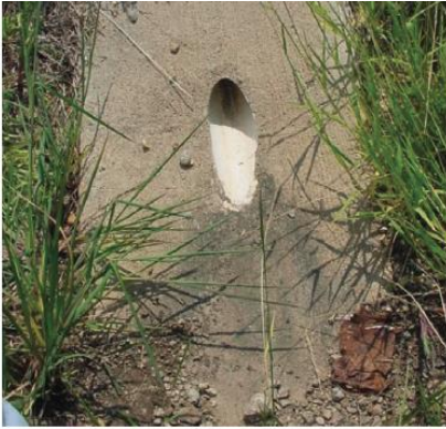
Figure 6. Rural subdrain outlet (Photo courtesy of Chapter 7, Concrete Pavement Preservation Guide, CP Tech Center)
