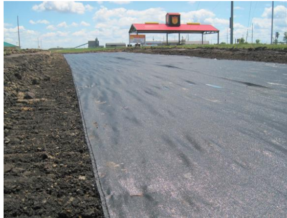
Figure 4. Woven geotextile placed in Boone County, Iowa (Boone County Expo research phase 1 – Granular road compaction and stabilization; InTrans project 12 – 433)
