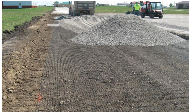
Figure 3. Rectangular geogrid placed in Boone County, Iowa (Boone County Expo research phase 1 – Granular road compaction and stabilization; InTrans project 12 – 433)
