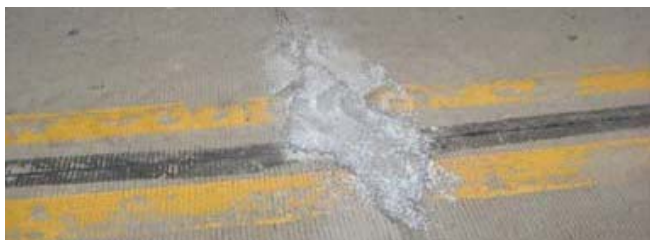
Figure 5-6. Pre-overlay repair of spalled joint (photo courtesy of Todd LaTorella, MO/KS ACPA)
