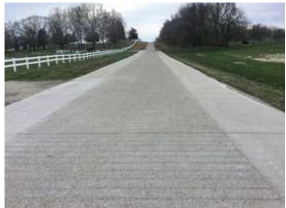
Figure 1-1. Eddyville, Iowa, cemetery road in spring 2016 (photo courtesy of Kevin Merryman, Iowa DOT)
