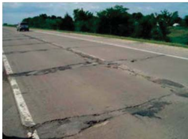
Figure 5-5. Concrete pavement with severe joint spalling (photo courtesy of Todd LaTorella, MO/KS ACPA)
