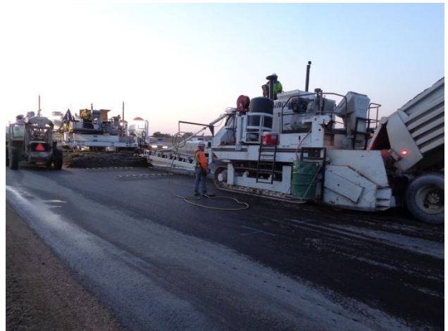
Figure 2. Trucks Dumping Concrete at Gomaco 9500 Placer, Installation of Dowel Baskets and Concrete Deposited Ahead of the Paver
