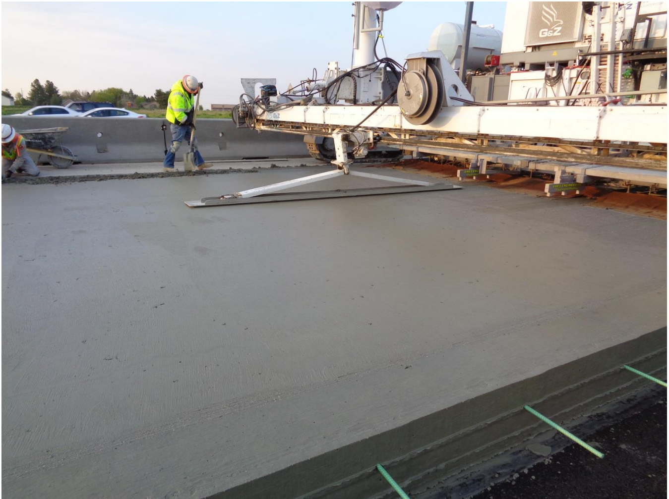
Figure 9. Nearly Vertical, Stable Slipformed Edge With Minimal Hand Finishing Required to Seal the Slab Surface
