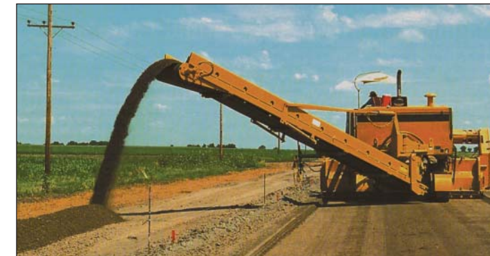
Figure 4. Autograder references the string line and trims the subgrade material (photo by American Concrete Pavement Association).
