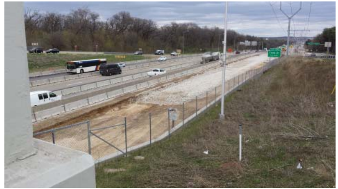
Figure 4. RCA spread for base course (Photo courtesy of Eleanor Bloom, Recycled Materials Resource Center)
