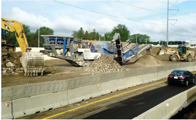
Figure 3. Onsite crushing operations at the Beltline Highway project (Photo courtesy of Steven Theisen, WisDOT)
